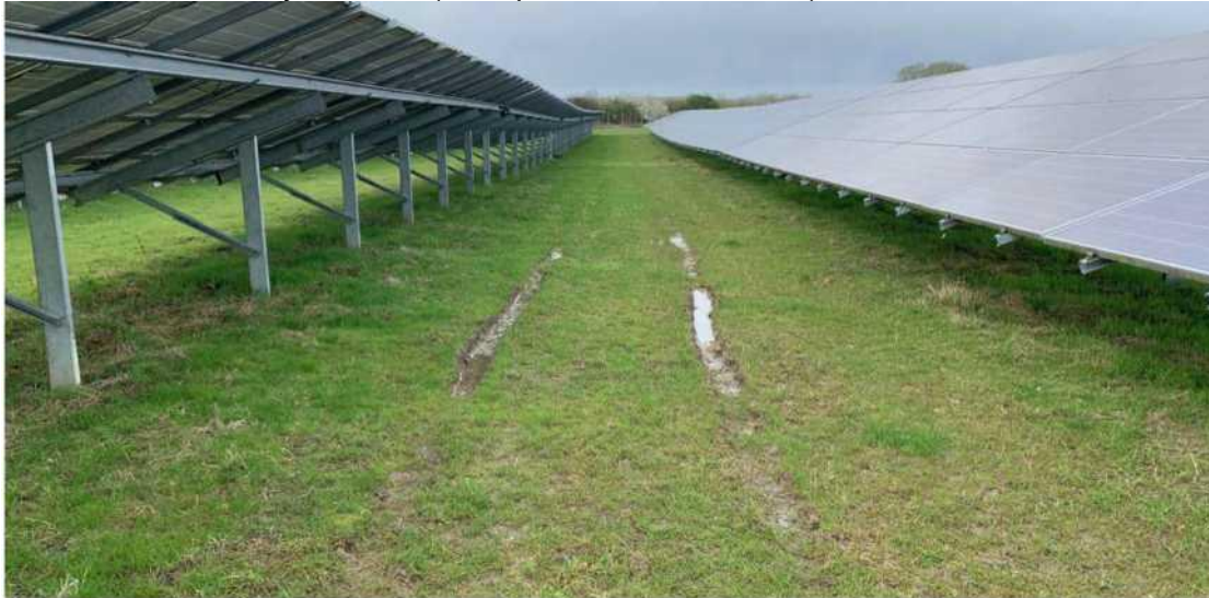
Insert 46: Ruts Caused by Vehicles (example from Staffordshire)
